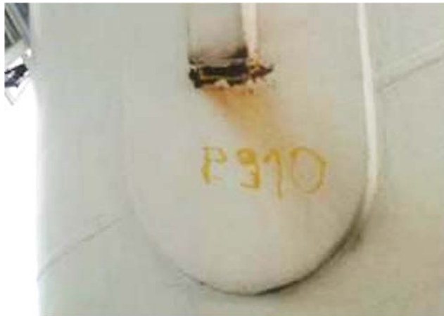
Figure 3: Cracking at the weld of the seal plate
