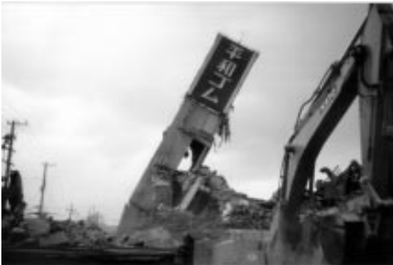
WEAK STRUCTURES FAILED
