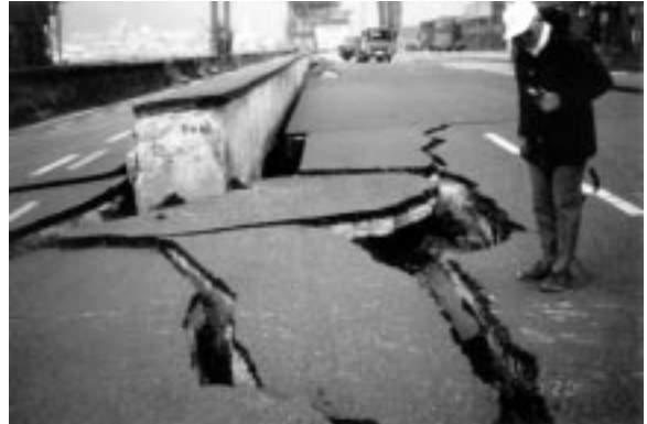
THE PAVEMENT SETTLED
