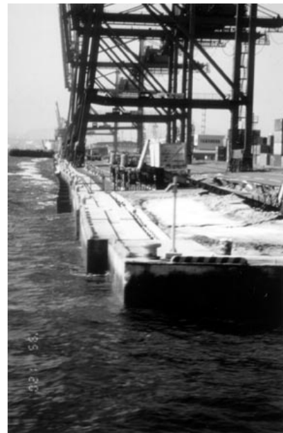
FAILED QUAY WALLS
