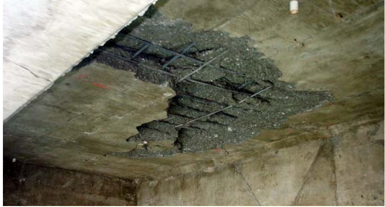
Punching and spalling failure – view from below wharf
