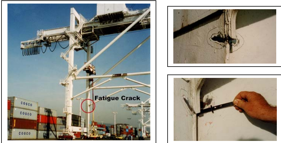
Oakland Leg Cracks
