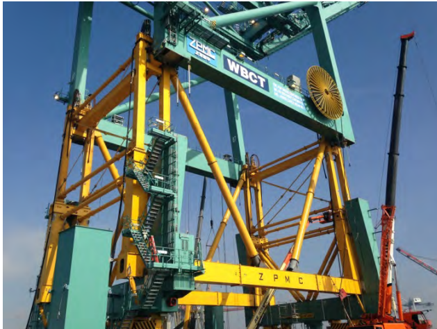
Photograph 2: Raised crane on jacking frame, with the new leg sections on the ground
